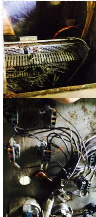
Above: Corrosion inside electrical cabinets. The insulation on the wiring has turned black, making fault-finding a long and tedious process which can add to machine downtime.
